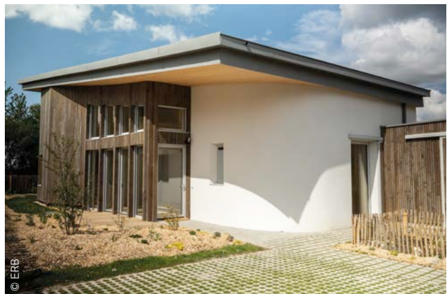
Fig. 20 Two 3D printed polyurethane foam walls between which concrete is poured (left); and the house called ' Empreinte ' (right).
