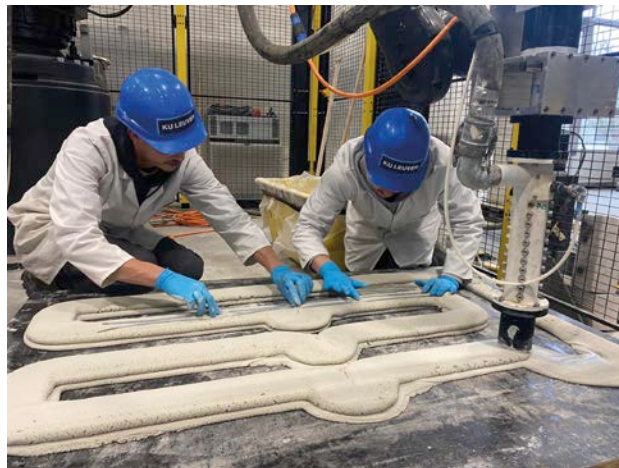
Fig. 22 Manually adding reinforcement between printed layers (element printed at Buildwise in collaboration with KU Leuven).
