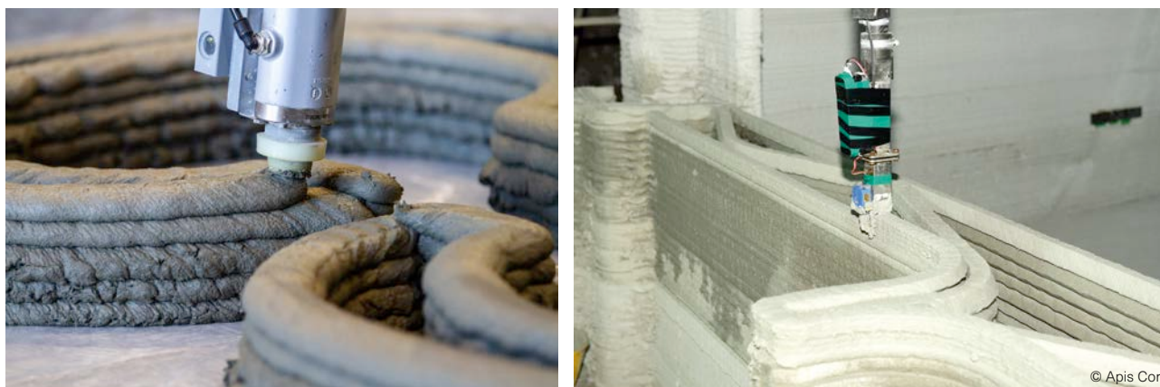
Fig. 33 Lateral layered surface (left) and using lateral trowels for smoothing the surface (right).
