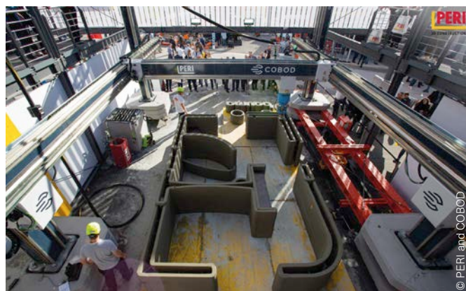
Fig. 35 3D printing the walls of a small house, outdoors, during the Bauma exhibition in Germany.
