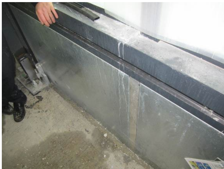
Figure 30 – E 60 fire-resistant facade element consisting of internal steel sheets (Lewven Fire Brigade).
